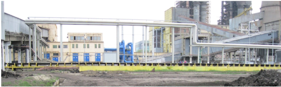
Fig 1. Belt conveyor for coal
